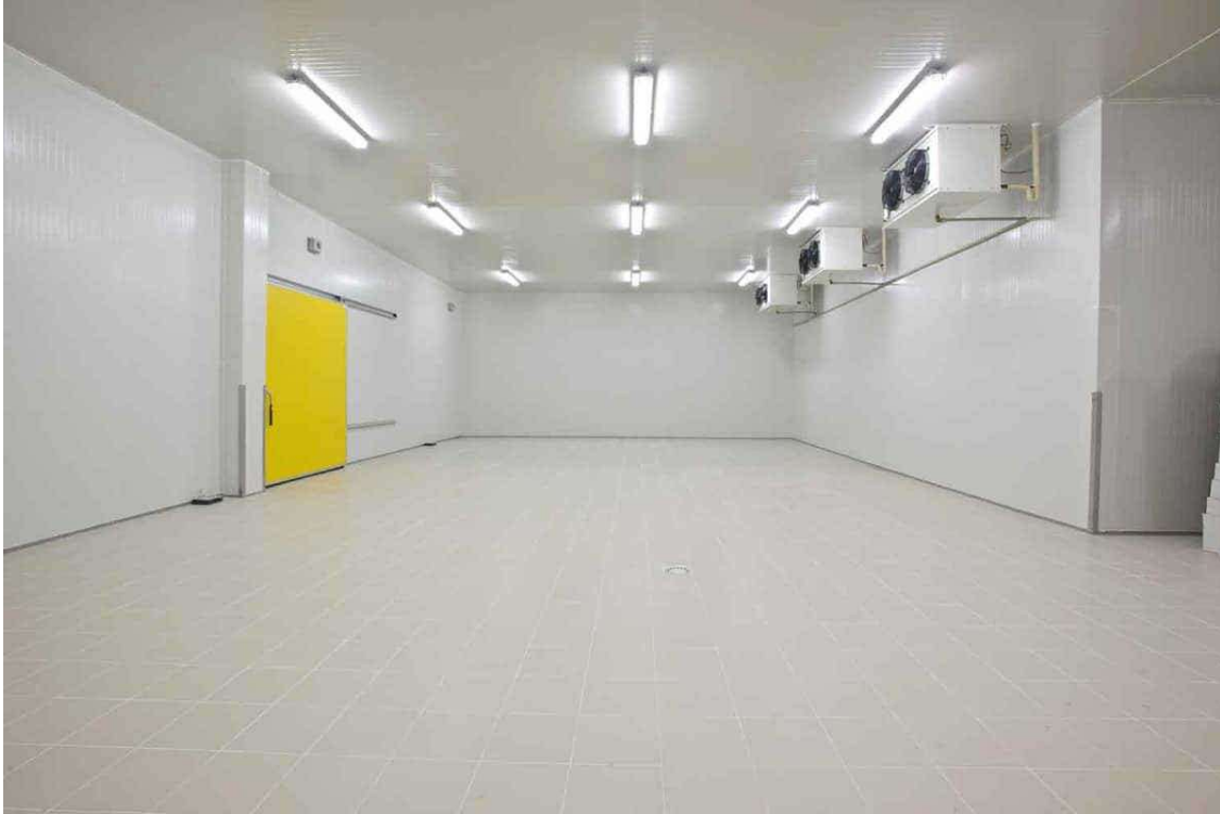
Figure 14. Cold Chamber. Source: Eletrofrigor (2006).
