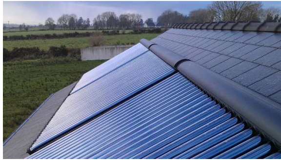
Figure 20 Thermal Solar Panels. Retrieved from: https://allianzenergy.com.co/capacitacion/energia-solar-termica/property-prices
