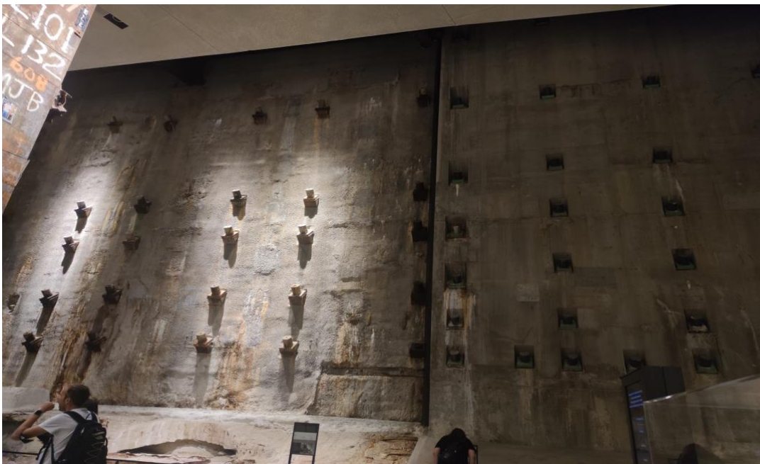
Figure 2. The Slurry Wall. Note. Image of the Slurry Wall taken from the Foundation Hall. (own photo).
