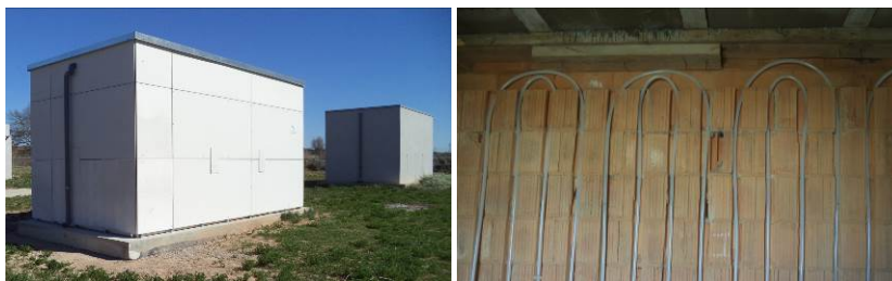
Figure 1: Radiant Wall cubicle and reference cubicle (left) and detail on installation of embedded pipes (right)
