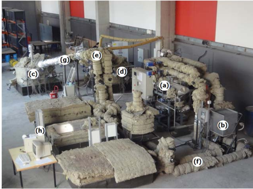
Figure 2. Overview of the pilot plant facility used to carry out the experimentation. (a) Electrical boiler, (b) Air-HTF heat exchanger, (c) Molten salts hot tank, (d) Molten salts cold tank, (e) HTF-molten salts heat exchanger, (f) HTF loop, (g) Molten salts loop and (h) Acquisition and recording system.
